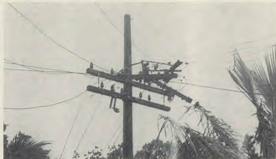
Why we had no power and no telephones for weeks. There were twenty-three miles of this kind of work to be done. (Photos this page: M. Porter.)
