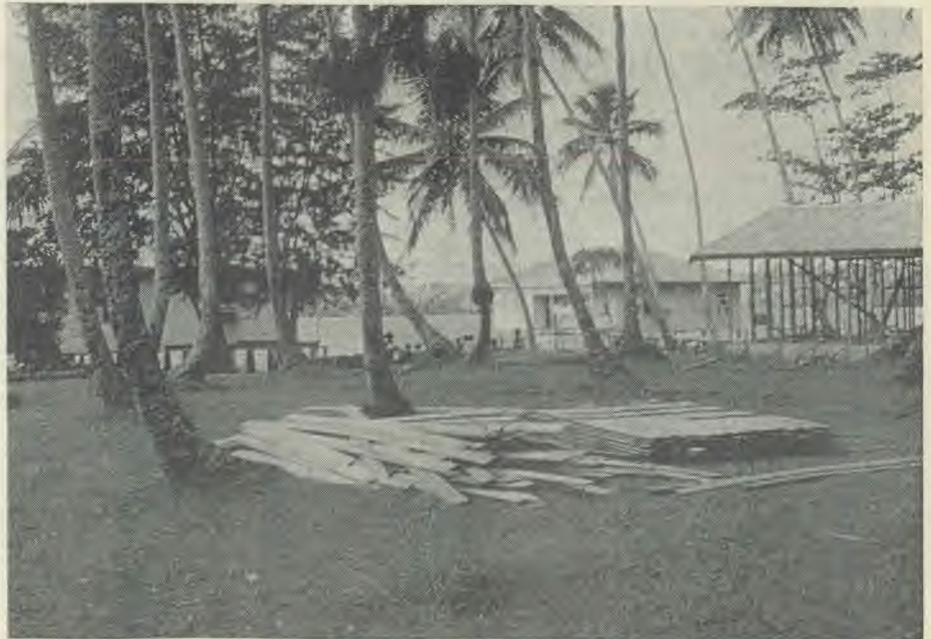
A pile of weatherboards for the new Batuna hospital, cut from timber supplied by the natives, waits for those things the natives cannot supply. The old hospital, to the left; the framework of the new, to the right. (Photo: Martin Brown.)
