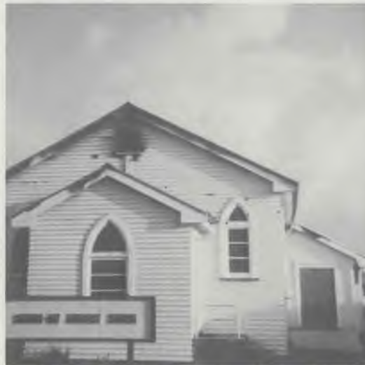
Betrayed by blackened roof—the fire-damaged Kaitaia church.
