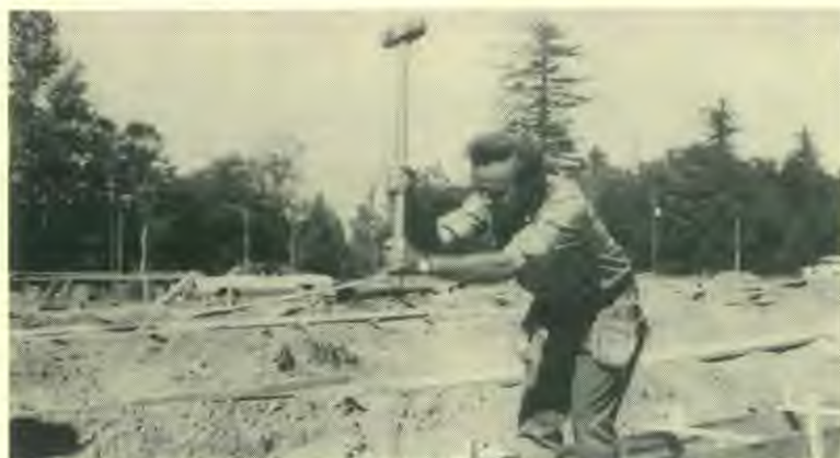
Construction foreman, Greg Eppel, places forms industriously and donates a full day's work each Sunday plus overtime.
