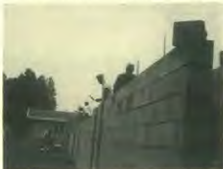
Workmen nearly lay school complex blocks in one week. Auditorium construction to follow when more funds become available.
