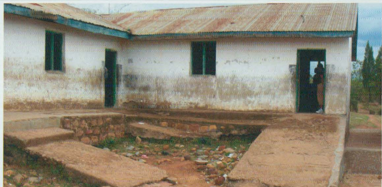
The Nyaburi School building is in need of renovation. New wheelchair ramps with railings are needed to meet safety standards and the leaky roof needs repair.
