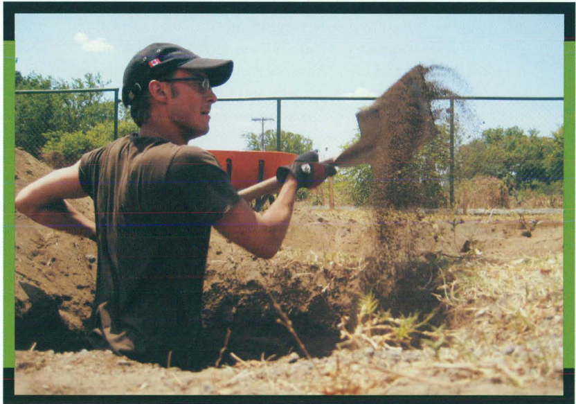
Remi Desjardins, a first-year Religious Studies major digging holes for the building foundation.
