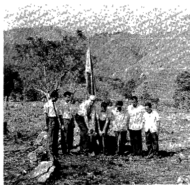
Pastor T. C. Murdoch (left with spade), Pastor H. E. McClure, and Mayor Magealeno Dazon of Tumbaga, Quirino, Ilocos Sur, breaking the ground for the Tirad View Academy on the foothills of Tumbaga Mountain. At the extreme left are E. L. Dingoasen, mission president, and Reuben Budayao, academy principal. To the right of the mayor are B. G. Mary, educational secretary of the North Philippine Union, and Magdalena Labagan, board chairman of the academy.
