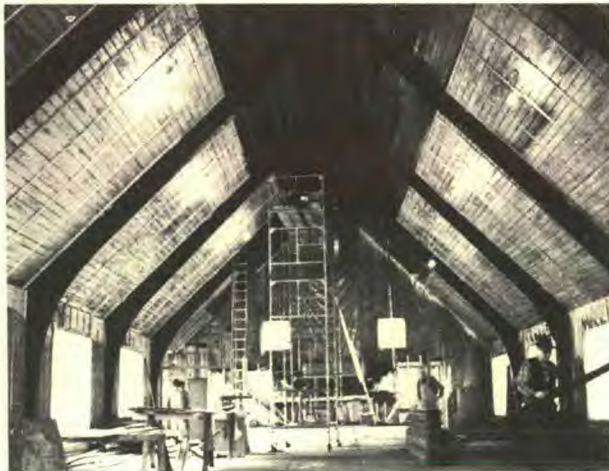
The interior of the Gary Glen Park Church is in the process of being restored.
