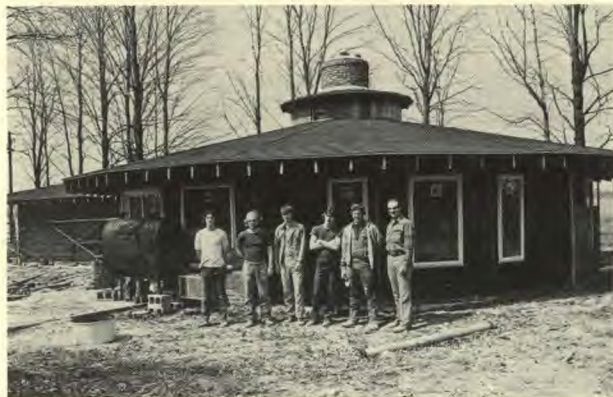
Occupational education students at the Andrews Center stand by the "round" house they are just completing. From left they are: Lloyd Draper, Eldon Jackson, Timothy Stockman, Dave Morford, Richard Brown, and director of the project, Farrell Gilliland, Sr.
