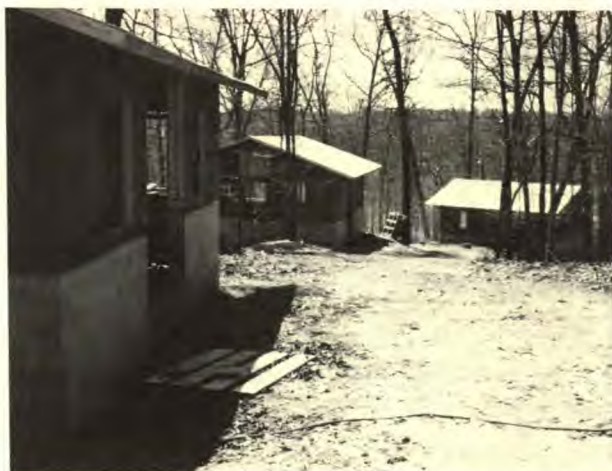
Here is a view of several new cabins under construction at Little Grassy Lake Camp.
