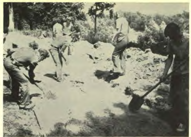
Students and staff work together to pour a concrete sidewalk in front of the administration building to connect the new boys' dorms.
