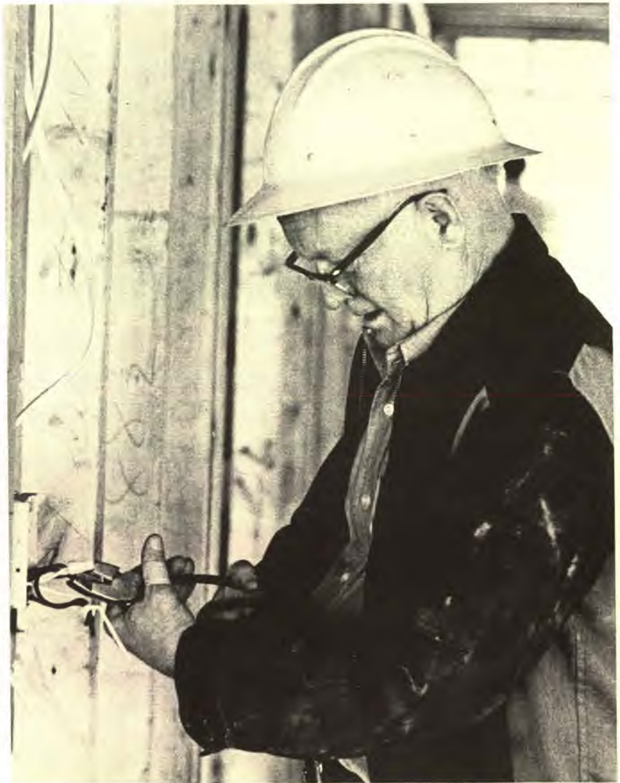
Bill Randall of Berrien Springs, Michigan, works with electrical installation on construction of the lodge at Valley Vista Center.
