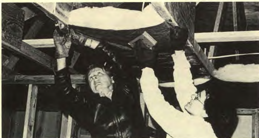
Mrs. Cloey Walls, left, of Bloomfield, Indiana, and Mrs. Mary Fleming, of Morgantown, West Virginia, install insulation material.
