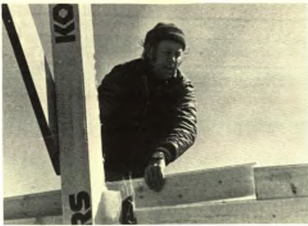
Local elder Chuck Morris puts a piece of roof decking in place.
