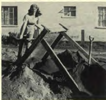
Sue Hart sifted sand for cement for the boys' dorm at Linda Vista.
