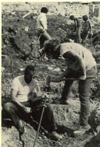
Allen First, left, and Dennis Meyers, right, dig a hole for dynamite to blast area for the sewage system at Linda Vista.
