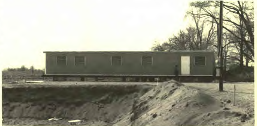
Excavation is complete on the site of the Athens Family Health Center property. The mobile office is being used in the interim until the completion of the family health center.
