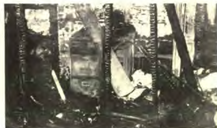
The pastor's study was heavily damaged.
