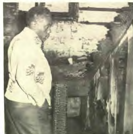
Charles Connor surveys interior foyer damage. Mr. Connor is chairman of the new church building fund committee.
