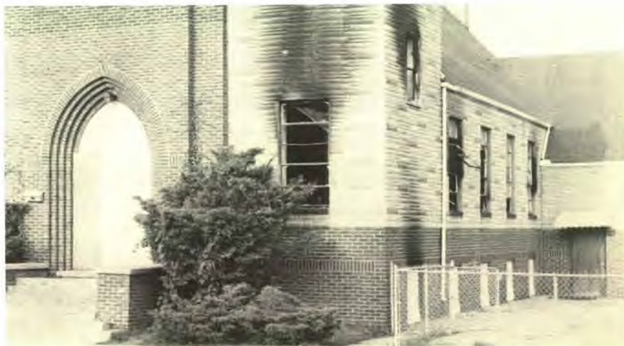
The fire left its mark on the outside of the church.
