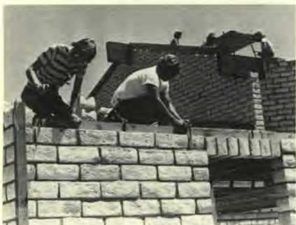
Dale Carothers, left, and Elwin Hutchins, right, apply roofing to the Vista Church.
