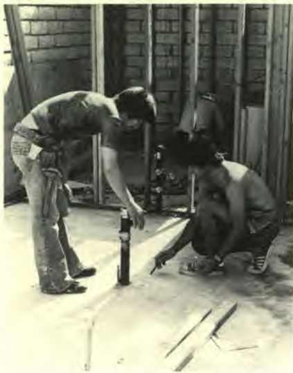
Mark Carpenter, left, and Bob Beck, right, confer on plumbing at the construction site in Vista.
