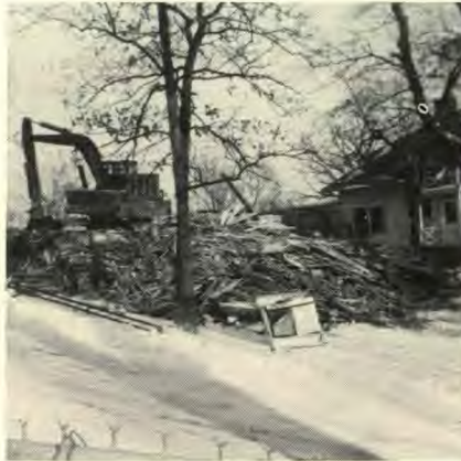
Only splinters remain as workmen clean up debris after the demolition of the former Wisconsin Conference office.
