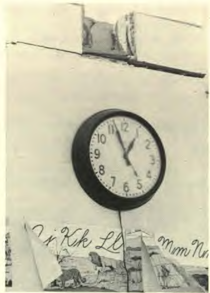
A large steel I-beam, 10 inches above the clock, was blown 200 feet across the highway.
