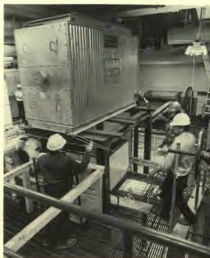
An economizer designed to reclaim escaping combustion heat was recently installed in Hinsdale Hospital's power plant. This is one of the first units to be installed in the suburban area.
