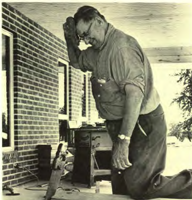
Ernie Reinhardt was the driving force behind the construction of the new Sheboygan, Wisconsin, Church. Photo courtesy of Sheboygan Press.
