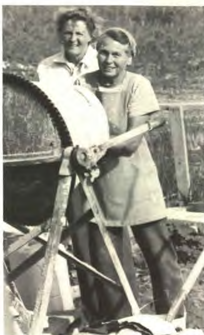
Myrtle Culp, right, and Bertie Jeffries, left, mixed mortar for the more than 2,000 blocks for the foundation.
