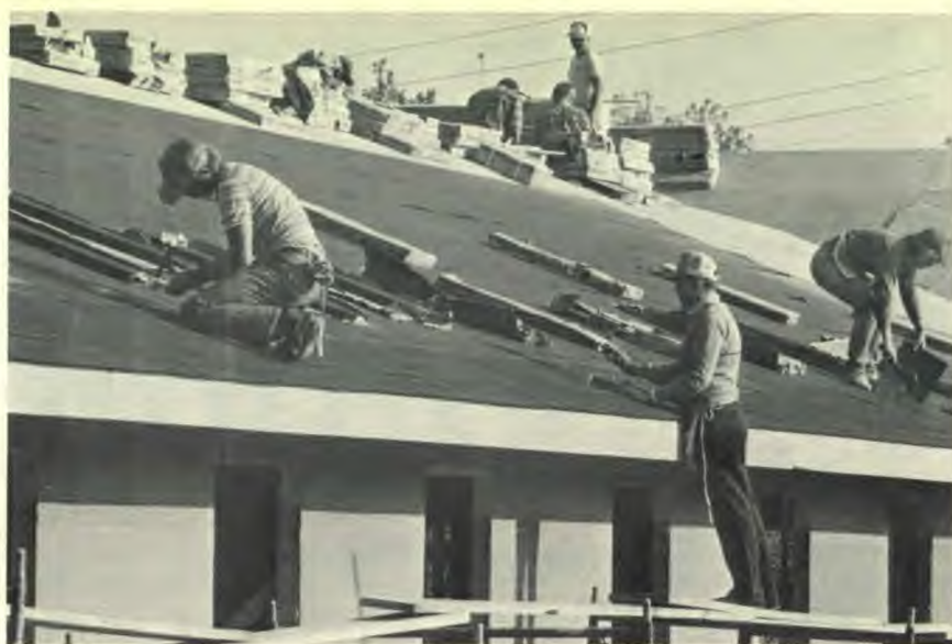
On a sunny day in late October volunteers shingled the new Glen Ellyn Church complex.
