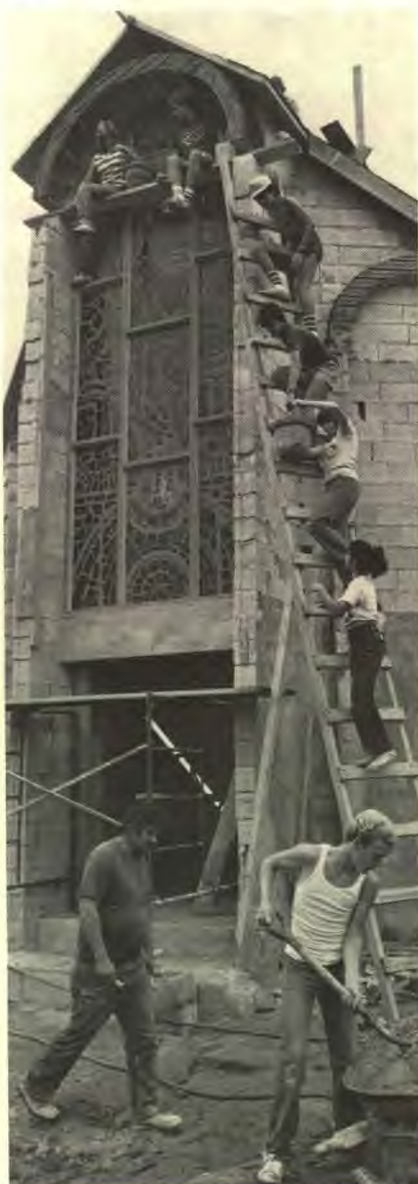
Mortar was carried by bucket to the roof peak of the church being constructed in Luquillo, Puerto Rico.
