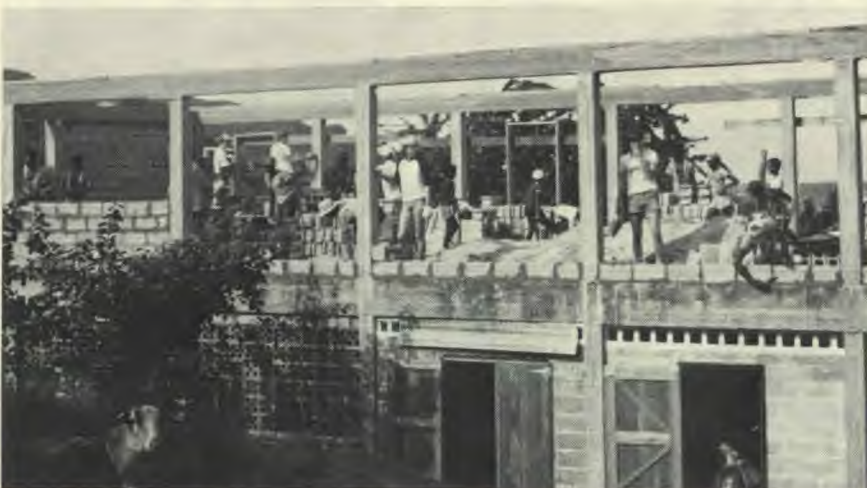
The second story addition to the Bequia school rapidly took shape and was nearly completed by the time students left.
