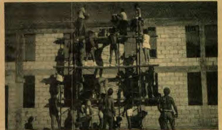
The gymnasium at Bahamas Academy as built by the Maranatha Flights International volunteers.
