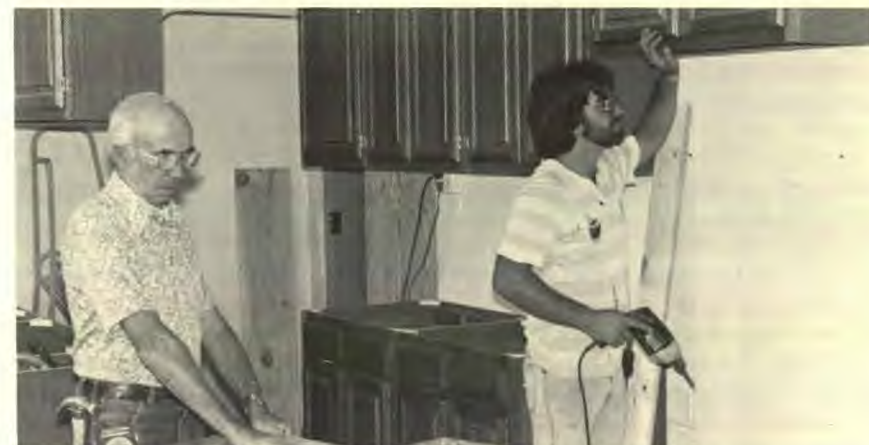
New cabinets were installed in the home economics room of the administration building.
