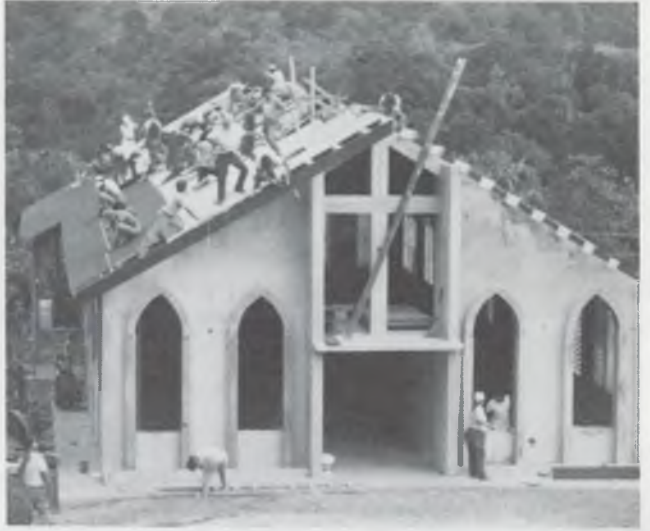
The roof was a busy place toward the end of the project as the students put the finishing touches on their efforts.
