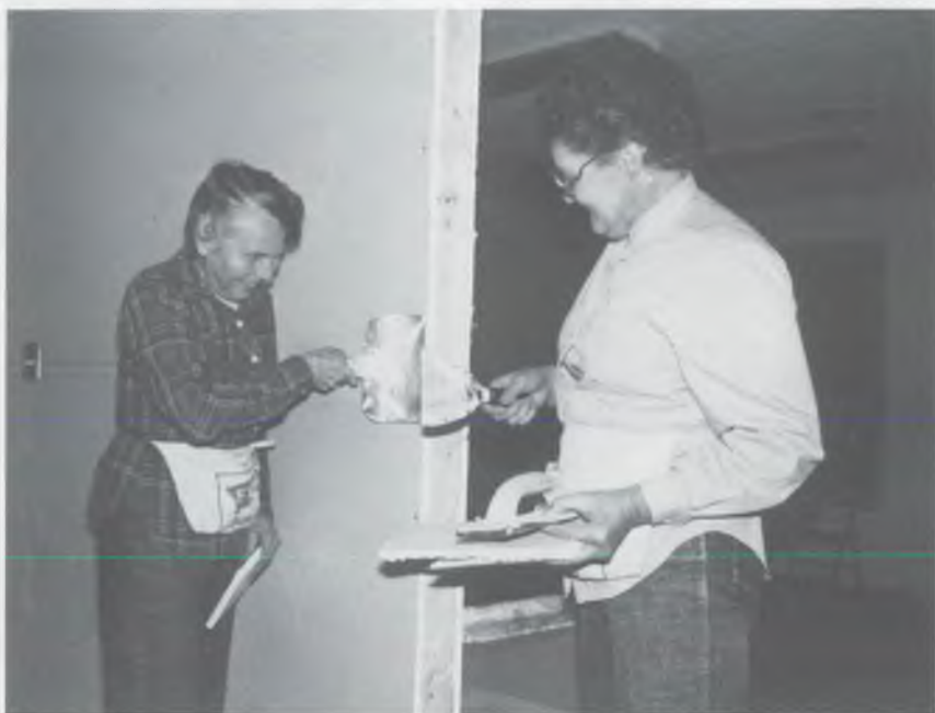
Myrtle Culp (left) and Bertie Jeffries demonstrate their dry-wall finishing skill in the new classrooms being framed in on the original plan.
