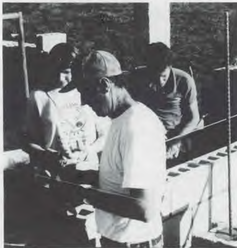
Steven Zmaj, a mason from Hartland Institute in Virginia, lays one of the 4,000 cement blocks to complete the second story project.
