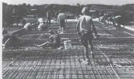
Before the roof could be poured, 1,250 reinforcing rods had to be put into place and tied.
