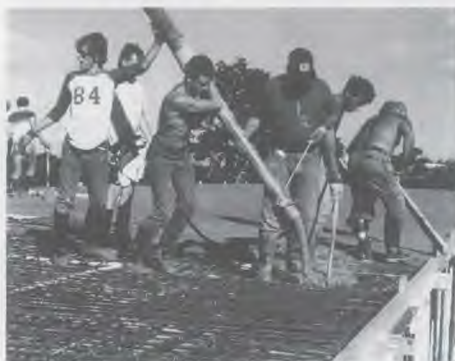
Some of the workers managed the cement pump while others troweled the surface of the roof.
