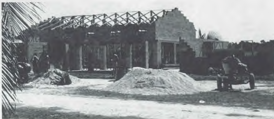
The Andrews group finished their work on Christmas morning by putting the roof trusses in place.
