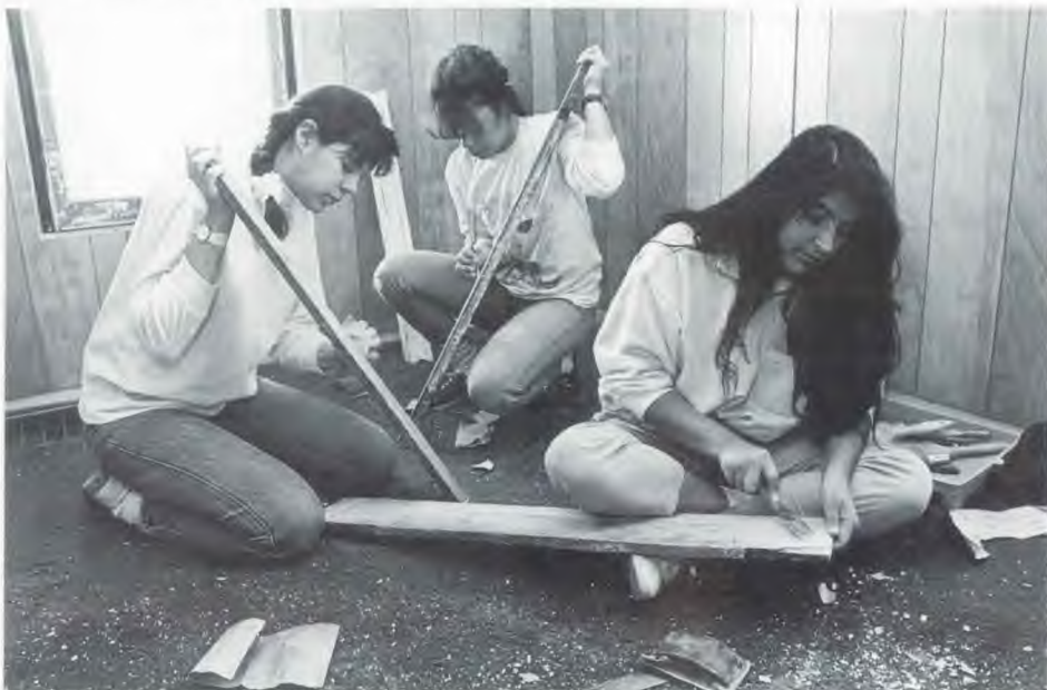
Stripping interior trim at the John Loughborough house are, from left, Yvette Vargas, Becky Figueroa and Miriam Verduzco of San Gabriel Academy in California.
