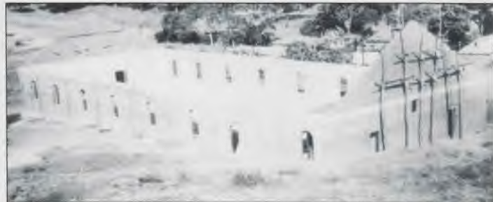
The Lilongwe Church is already under construction as the Eastern Africa Division anticipates the special offering on December 28.
