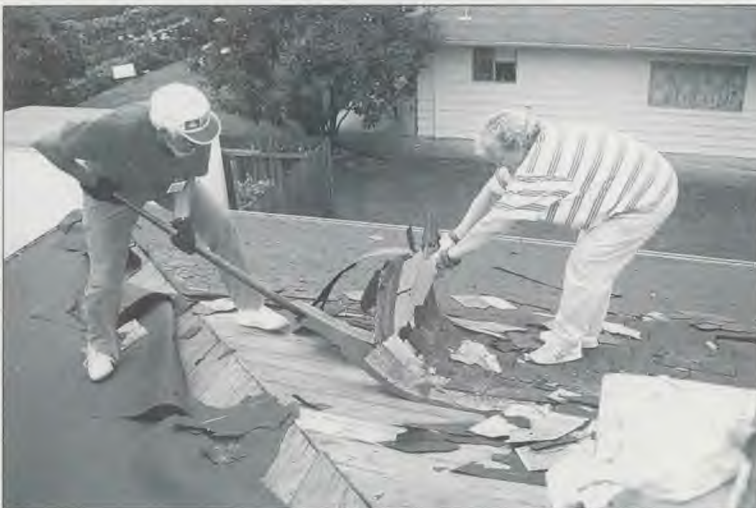
One hundred ten people worked for two weeks prior to the Maranatha Convention, July 29-31, renovating and re-roofing seven faculty homes, as well as remodeling the Auburn (WA) Academy administration building.
