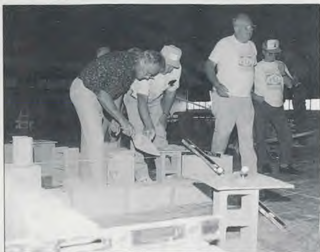
Maranatha volunteers learn the basics of laying cement blocks at the Friday afternoon seminar, "Lay A Brick For God."
