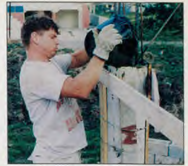
Jay Preece of Rockford, IL, carried cement in a bucket and hand-poured it into column forms. Jay was part of 19 volunteers from Illinois, Michigan, Minnesota and Wisconsin who worked on the school Dec. 8-22, 1993.
