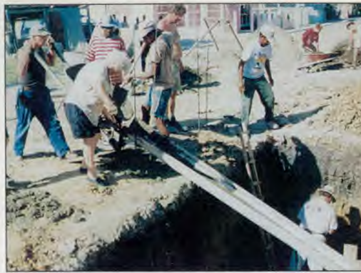
Volunteers from Wisconsin pour concrete for the floor of the cistern in December 1993.
