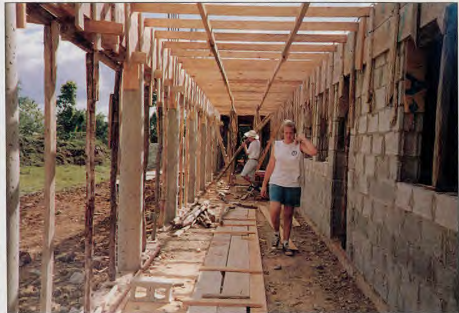
Seventeen members from two Berrien Springs (MI) churches went to help in December 1993. They completed the structure of this front porch.
