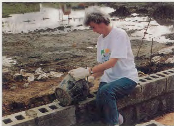
ASI member Betty Harris of Spruce, MI, grouts (fills holes) in the block walls of the new church school. The structure, when completed, will be 156'8" x 28'8" and contain five classrooms, two bathrooms, and two offices.
