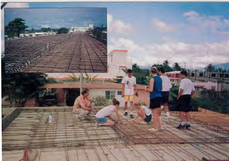
Berrien Springs members tied concrete reinforcing bar on the roof. It took the 17-member crew 64 hours to complete this job.
