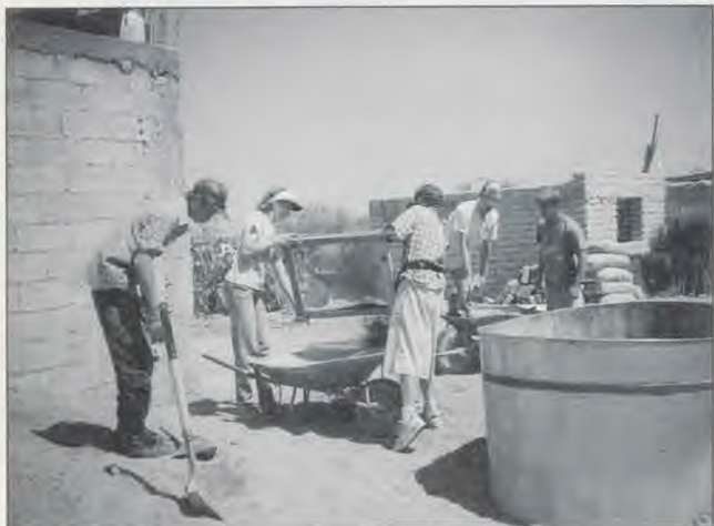
Wisconsin members work at a church site in Huizache, Mexico ("a wide spot in the road on the Pan American Highway").
