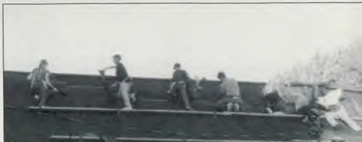
Indiana Academy students and various church members work to replace the roof of the Vincennes (IN) Church.
