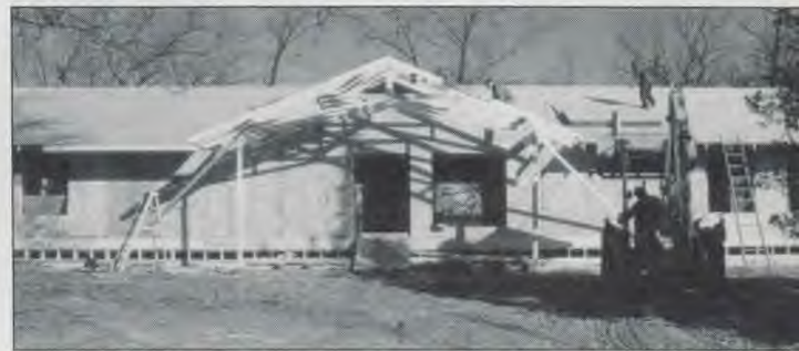
Both lodges' walls were up and the roofs ready for shingles by mid-November 1994. Roughly 45 volunteers got the majority of the work done during a two-week fall framing bee.
