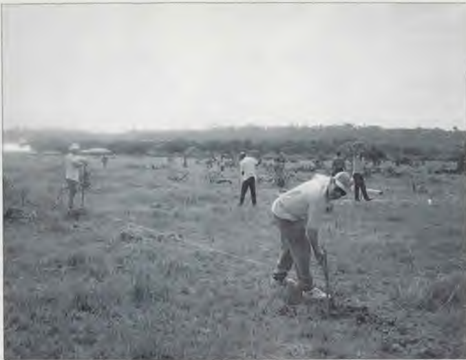
Starting "from scratch" the site had to be prepared. Stevensville members, Randy Dowell and Jim Hippler begin digging the post holes.
