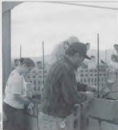
Jim Hippler, construction superintendent, teaches Andrews Academy students the art of block-laying their first day on the Puebla Nueva Church project in Agua Prieta, Mexico.
