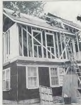
South Haven Church members came to the aid of the Schmeling family by closing off a new addition and roof before the rain came.
