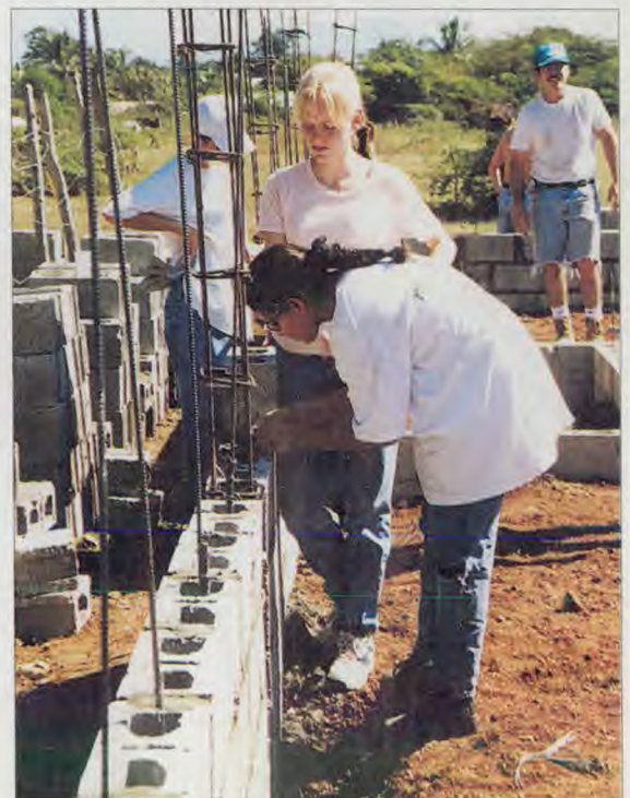
No sissies, the girls work right along with the guys on the construction site to help complete the job.
