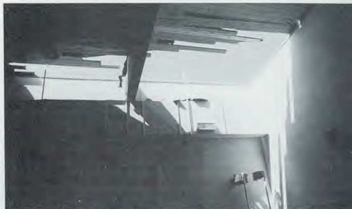
Daylight shines through the holes in the gym roof the morning after the storm. Graduation ceremonies had to be moved to the chapel in the administration building.
