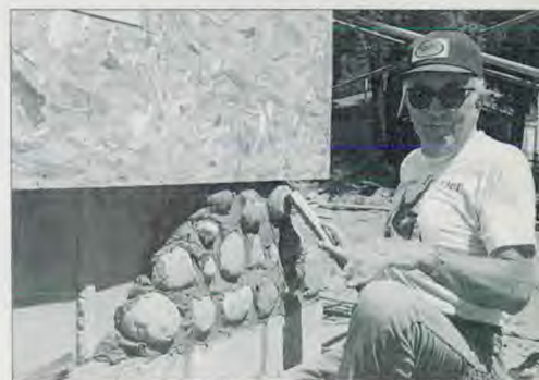
Ralph Benedict, a Battle Creek resident, works with rocks and mortar to simulate the foundation of the meetinghouse.
