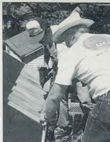
Joe Tweedy, from Eagle Bend, Minn., staples cedar shingles to the roof, assisted by Ed Harlan from Charlotte, Mich.
