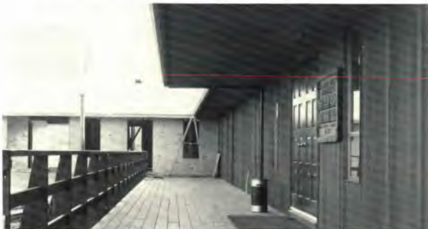
Additional offices are under construction in the professional office building next to the hospital.
