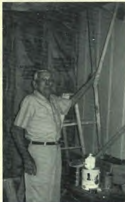
Earle Afton helping the carpenter install sheetrock in the porch of his home.
