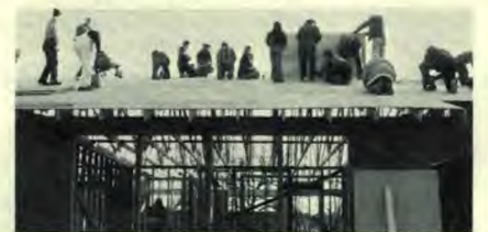
Beginning at the concrete foundation with only the plumbing in, Maranatha workers completed the framing and roof sheeting of the Junction City Church Sabbath School wing in one day.
