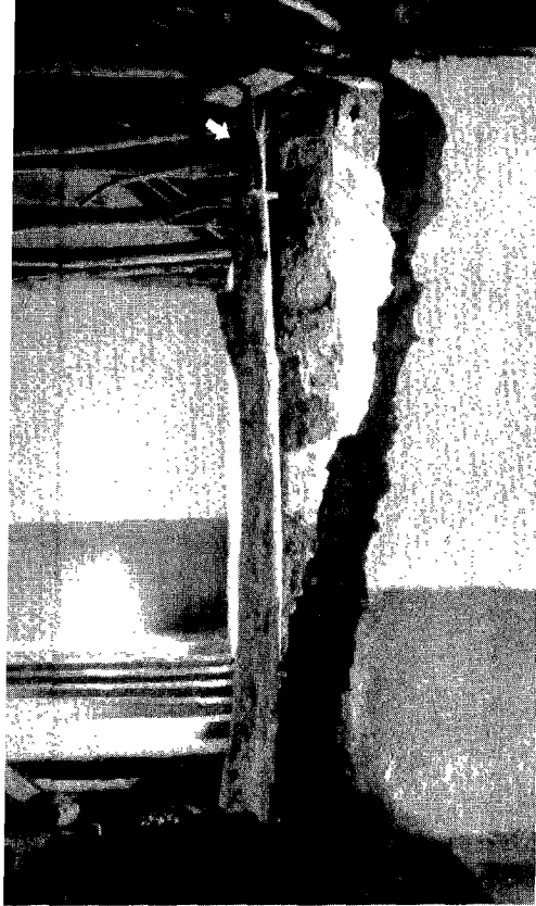
The Hanke Mission Station church in Rhodesia, showing the mission director's automobile jack (arrow) supporting the roof.
