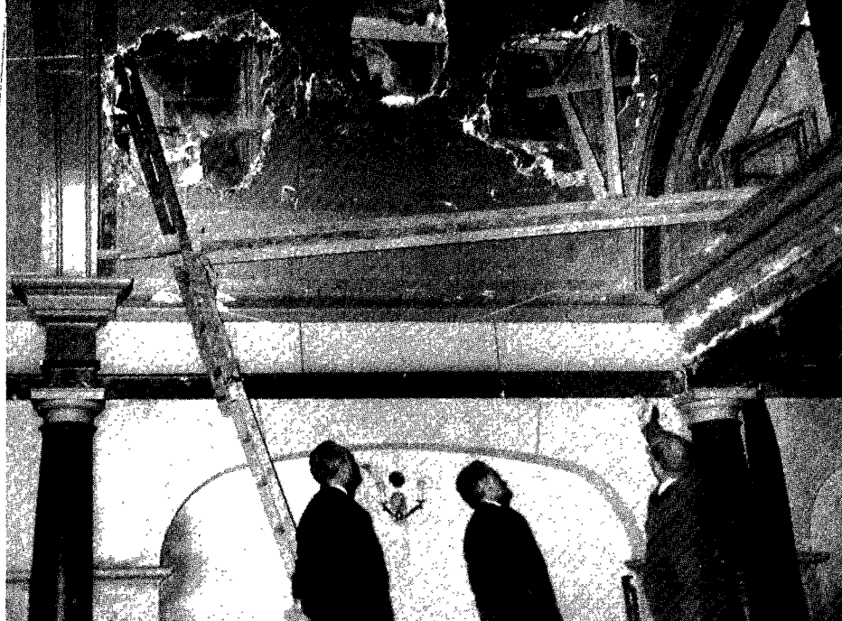
Pastor Antonio Bueno points to damage done by rain in the Madrid church while Alvaro Martin, treasurer (left), and Angel Codejon, president of the Spanish Mission, look on.
