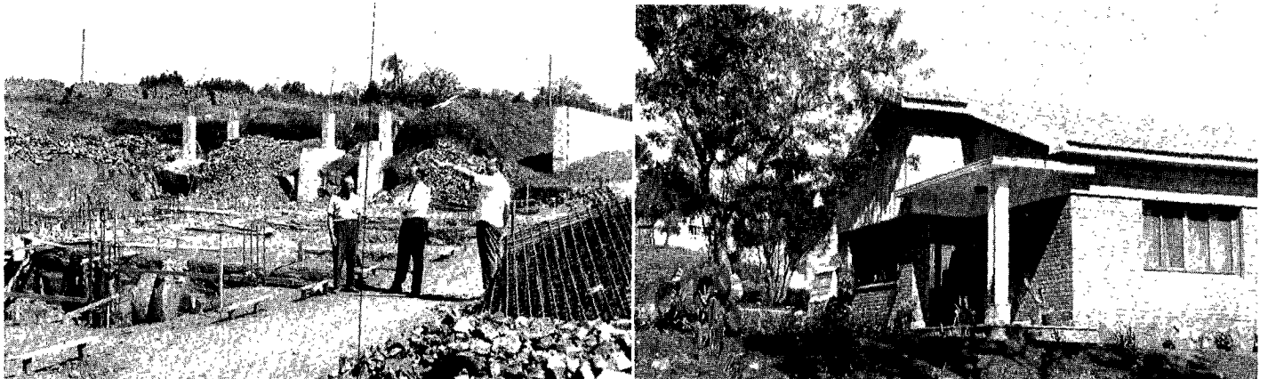
Left: Foundations are in for a new sanitarium in Misiones Province of northern Argentina. Inspecting the site are the builder (left), Austral Union president Elbio Pereyra, and manager Romualdo Kalbermatter. The building's 91 supporting columns are sunk 27½ inches in solid rock. Right: Two comfortable houses for doctors, like this one, have already been completed at the site of the new sanitarium.
