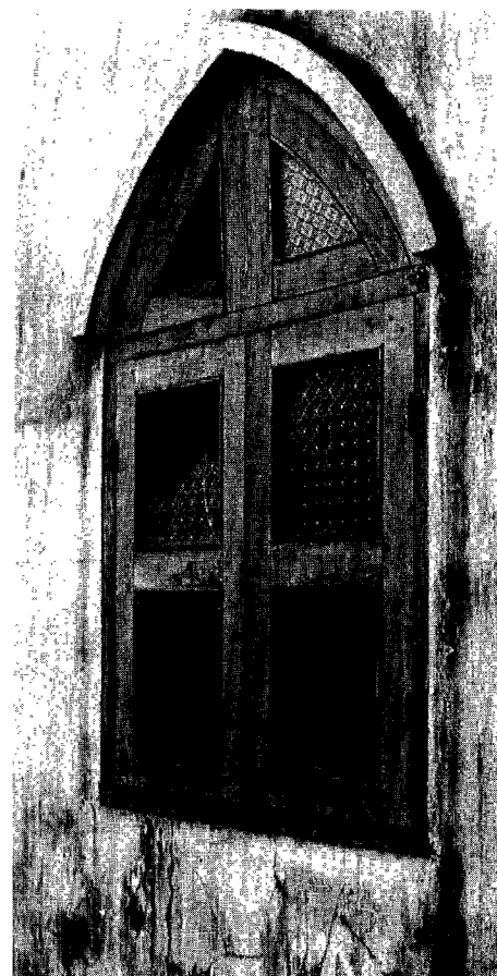
Damage such as this broken window, created during one of several war skirmishes in the vicinity, forced the closing of the Bienhoa church for the past two years. Having been situated in a shell-riddled war zone for the past six years, the small church has had its windows broken and wooden frames for both doors and windows destroyed. The church is now planning to open again since conditions have become more peaceful in this area a few miles northeast of Saigon.
