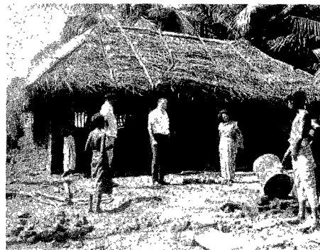
A new home is being built in the flood-ravaged area of Ceylon by relief funds. Lawton Lowe, president of Ceylon Union, who stands between Kingsley Peter, pastor of the Galle, Ceylon, church, and Pastor Peter's wife, inspects the new structure.
