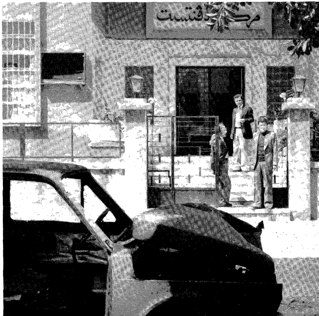
Apart from shattered windows, the Beirut Evangelistic Centre shows no signs of having been struck by a rocket on the night of March 23. Ernest Runge, looking through the broken glass, secures the building against intruders as Alfred Brandt, Milad Modad, and Borge Schantz, on the steps, discuss the night's happenings.
