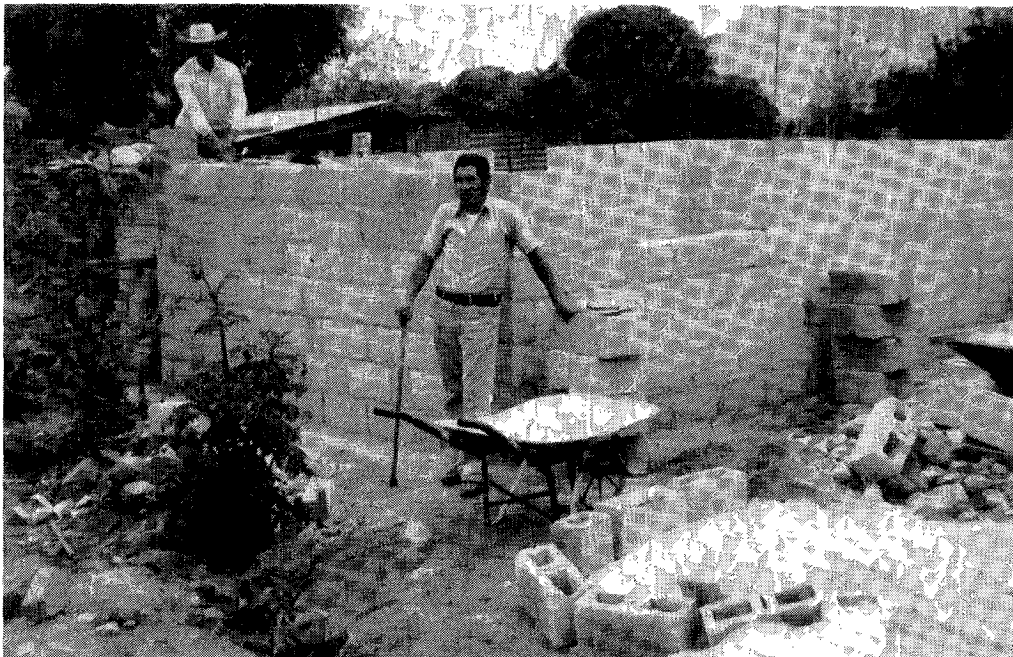
Review readers provided funds for Mr. Oswaldo's new home, which is being built on the spot where his two daughters lost their lives in the Guatemalan earthquake. Mr. Oswaldo walks with a cane and wears a brace because his back was broken by falling debris during the earthquake. Forty homes like his are finished now.
