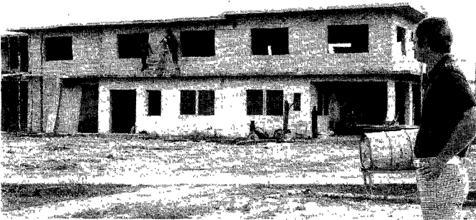
Top: A Quonset hut formerly was the girls' dormitory at Palau Mission Academy, but now the girls live in a building constructed last summer (bottom) by volunteers from the U.S.A. Church members raised the money to complete the project, begun with Thirteenth Sabbath Offering funds.
